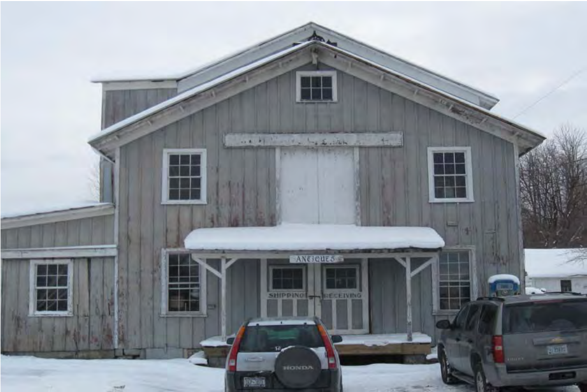
Photograph 2. View of the front of the mill building/former electroplating facility along Green Street. View to the south.
