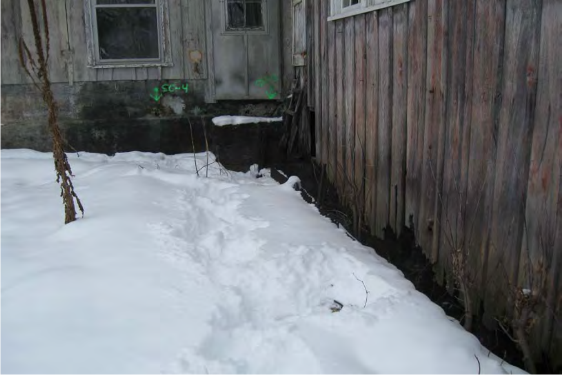
Photograph 9. Detail of in situ iron trash racks, seen jutting above the snow at the center of the photograph, at the base of the mill extension (section “K” in Figure 4”).
