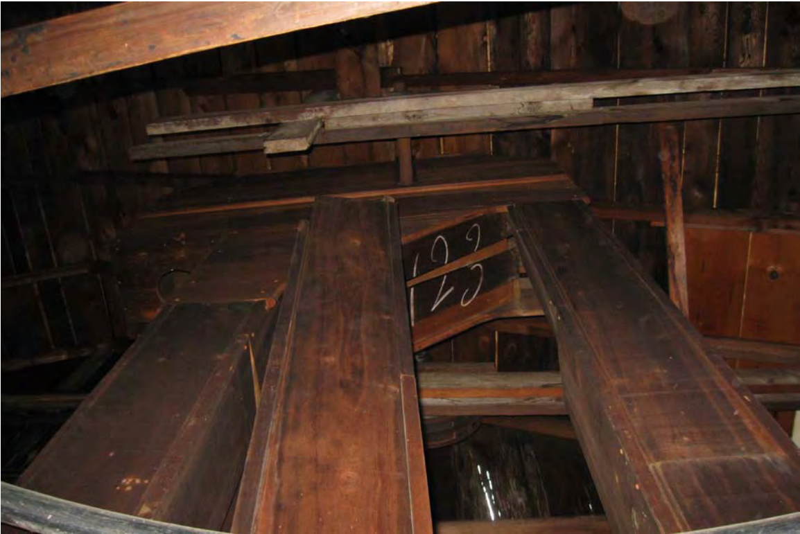
Photograph 10. Detail of intact box conveyors used for transporting grain through the mill (located in section “I” in Figure 4).
