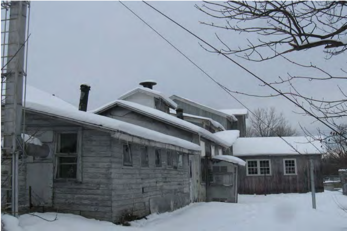
Photograph 6. View of the rear of the mill building/former electroplating facility. The sheet-metal smokestack provided draft for a boiler and later furnace. View to the northwest.
