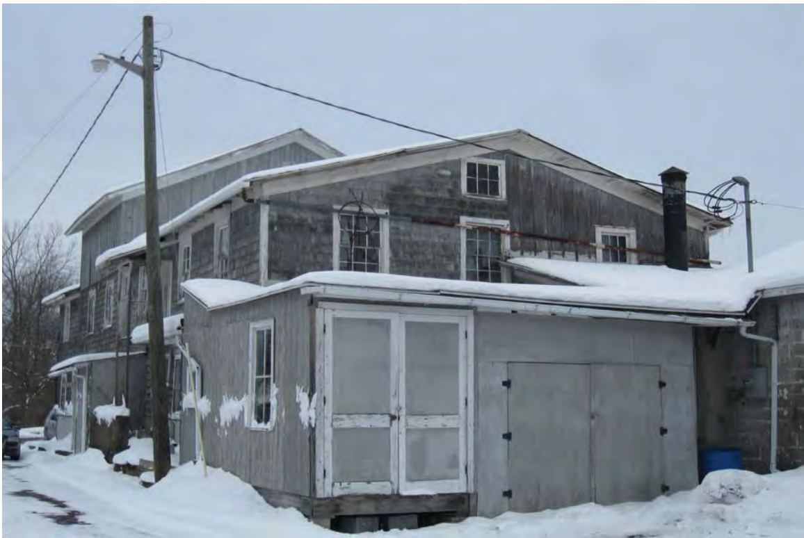
Photograph 4. View of the rear of the mill building/former electroplating facility. View to the north.
